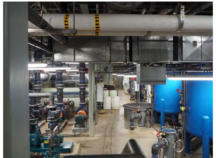
General view of WEA mechanical room (from IE tour in November)
