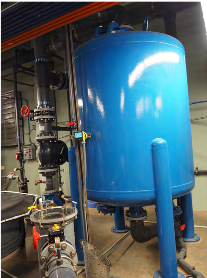
Huge blue canisters are sand filtration tanks (from IE tour in November)
